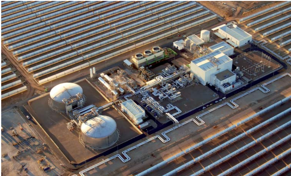
Figure 8. BOP and storage system of the power plant La Florida in Badajoz. Owned by Renovables SAMCA.
