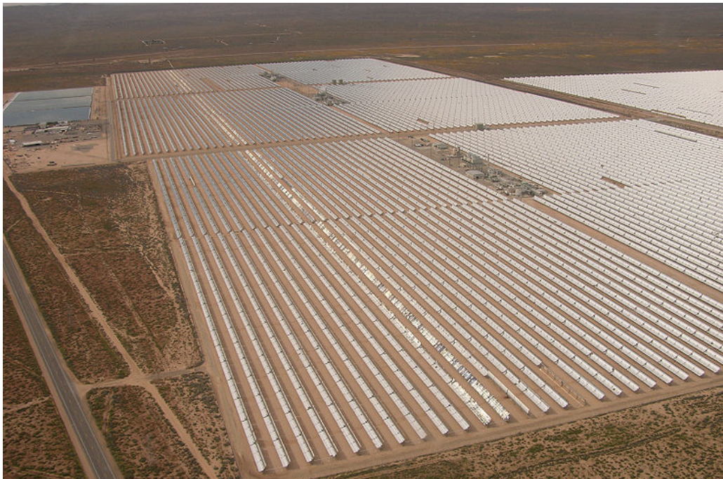
Solar Energy Generating System (SEGS), Kramer Junction, California, USA (354MW) – operating since 1986
