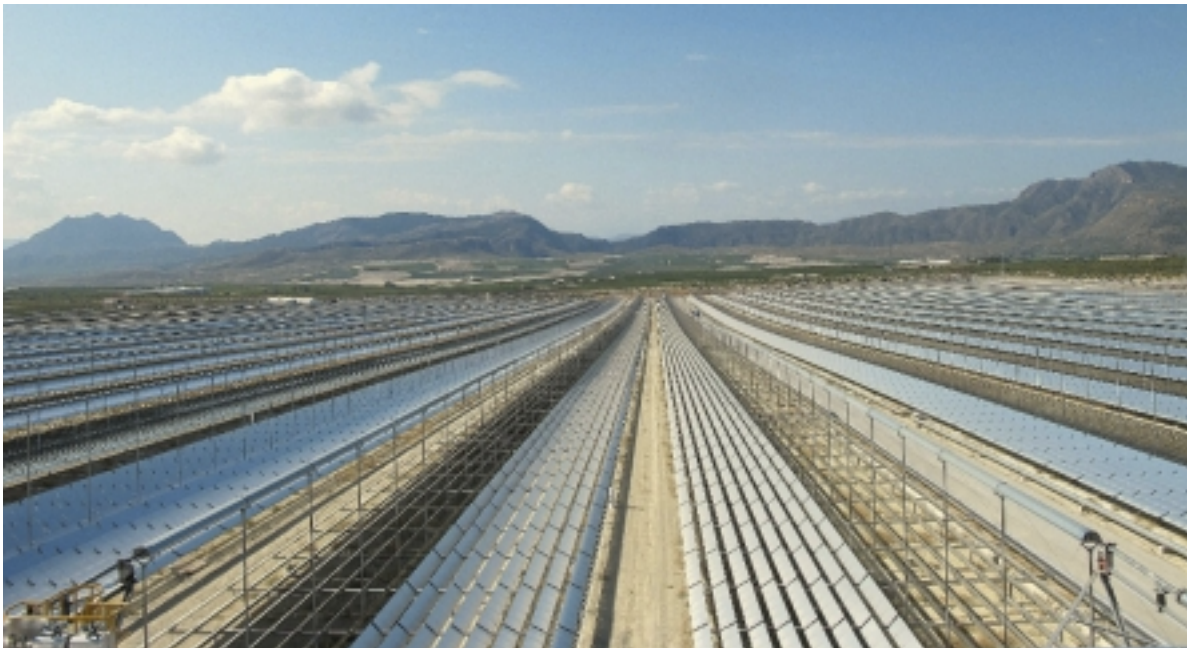
Novatec Solar – Puerta Errado 2 (PE2) Linear Fresnel Power Station Calasparra, Murca, Spain (under construction)
